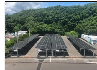
the solar power generators on the carports
