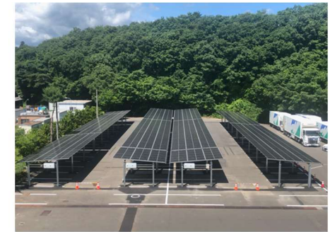
Solar panels on the carports for employees
