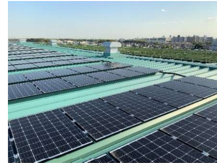
Solar panels on the rooftop of facilities
