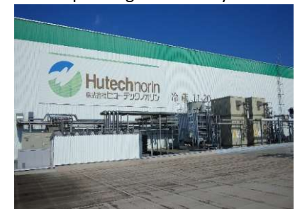
Installed refrigerators with natural refrigerants
